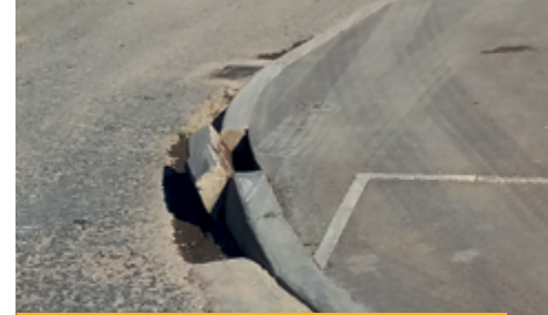
Prevent kerb damage
